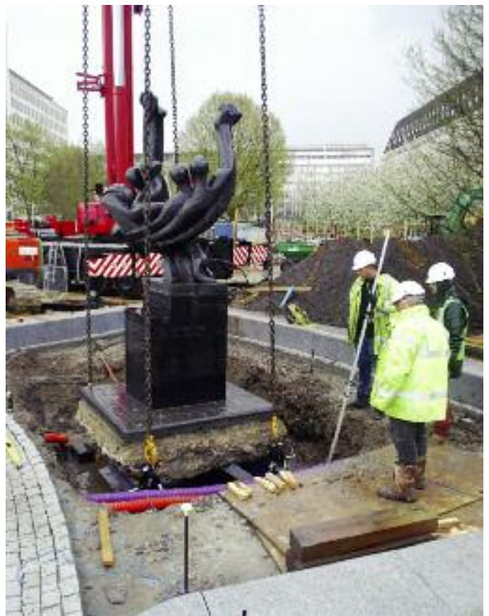
GROUNDING: A crane manoeuvres the 9-ton International Brigade memorial and base to its new position in London’s Jubilee Gardens on 19 April.
